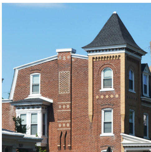
Chimneys with decorative brick coursing are distinctive and should be preserved even when capped and no longer in use.
