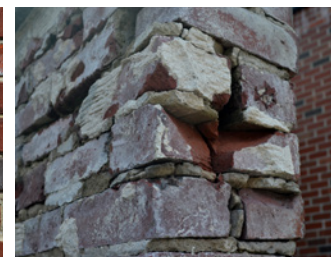
Mortar is incompatible with historic masonry when it is too hard and causes brick spalling and breakage.
