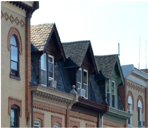
Three roofs show the visual differences in roof materials: original slate (left), 3-tab asphalt shingle (center), and variegated-width architectural shingle (right).
