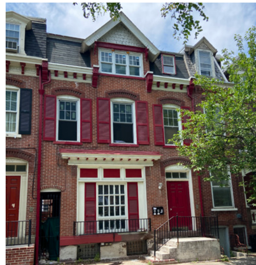
The drainage system shared by these two rowhouses has been painted to blend in with the rest of the building details. Downspouts connect to each building's built-in box gutter.
