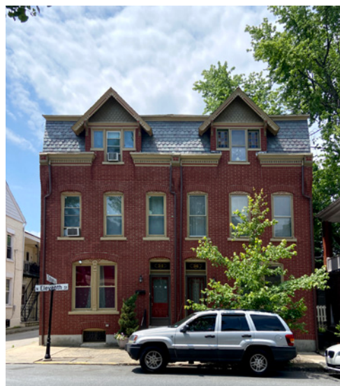
Dormers are integral parts of both a roof and a decorative scheme. Original trim, cladding, windows, and roof materials should be preserved.
