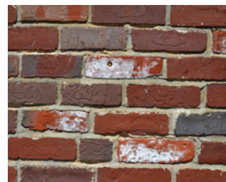
Efflorescence is a white haze caused by the migration of salts through masonry units.
