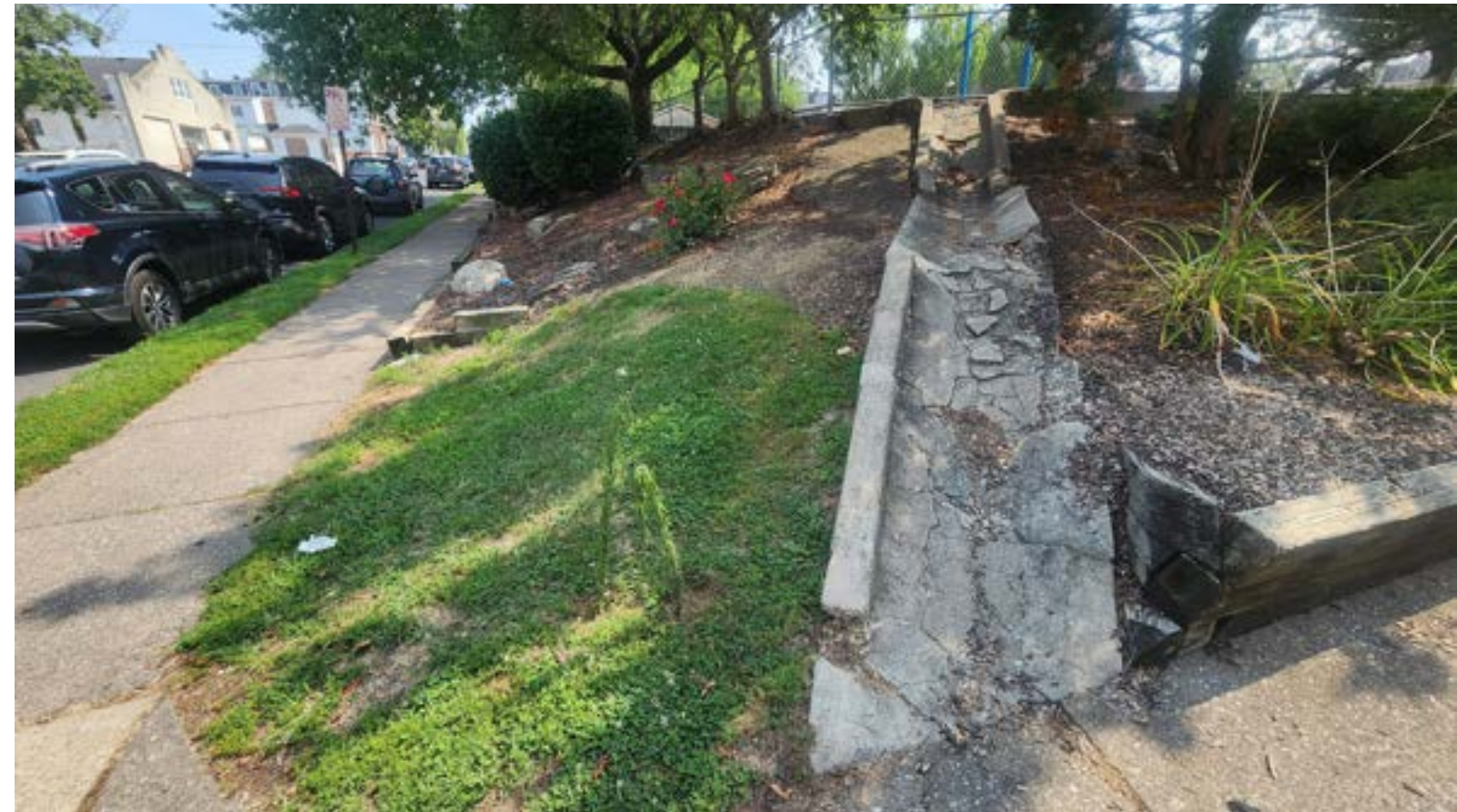
Stormwater is conveyed off of Franklin Park and into the streets by way of this deteriorated runnel system.
