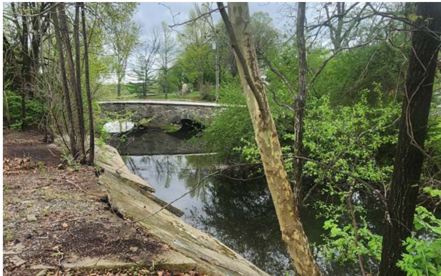
Dislodged, obsolete concrete slab embankment armoring threaten the historic Walnut St Bridge. City-partnership investments to solve these erosion/floodplain issues are essential to protect MLK Trail improvements to be installed directly downstream through Union Terrace Park.
