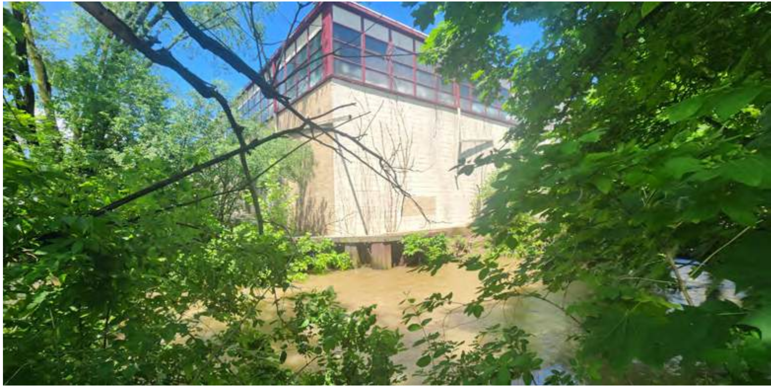
Derelict building constructed into Cedar Creek
