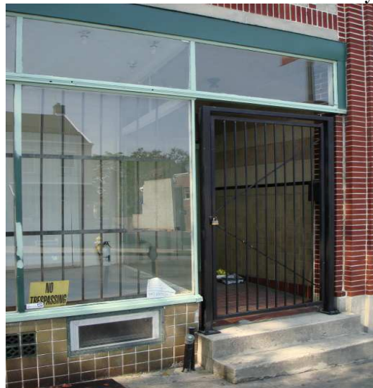
Inappropriate Security Grille
