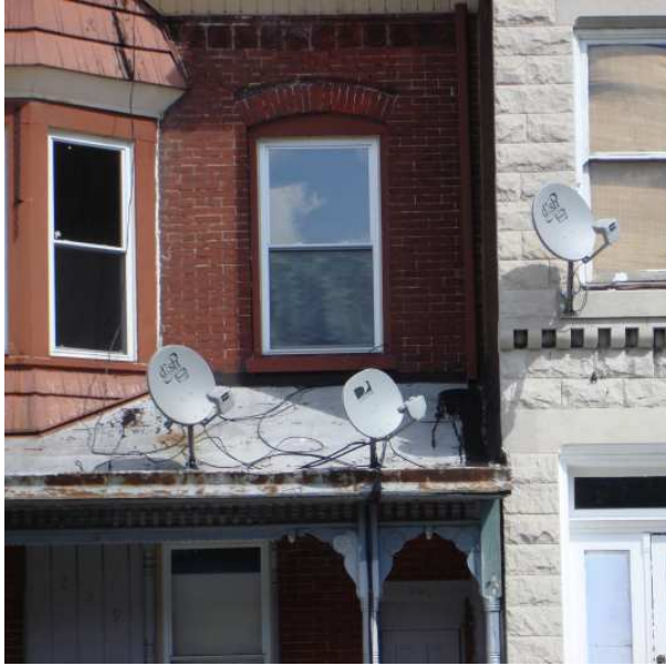
Inappropriate Façade Elements
